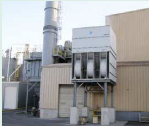
WFI's closed-loop water cooling system.
