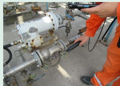
Detecting a VOC leak.
